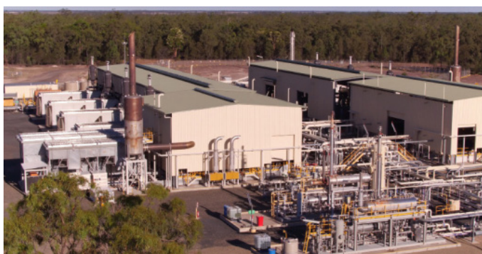
Daandine Power Station
